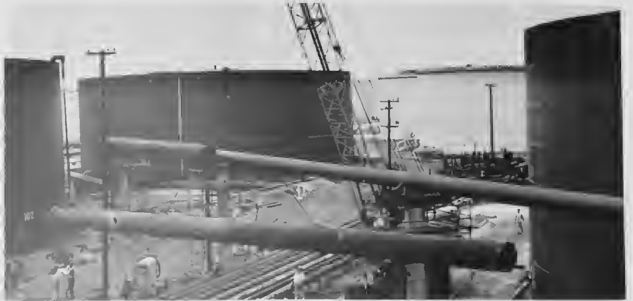
THIS SCENE in the tank farm shows the dimensions of pipe sections as a crane swings them into place. For the longer pieces, two 44-foot sections were welded together before being mounted.
